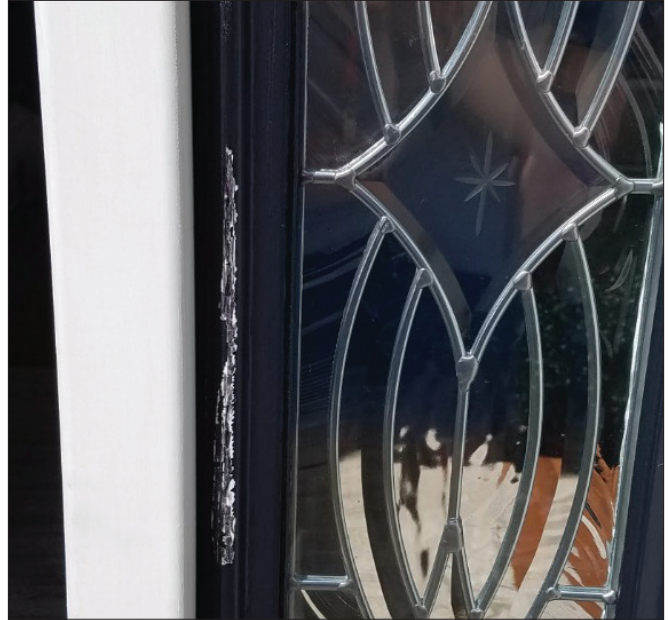
Paint Issue not easily serviced in the Field
